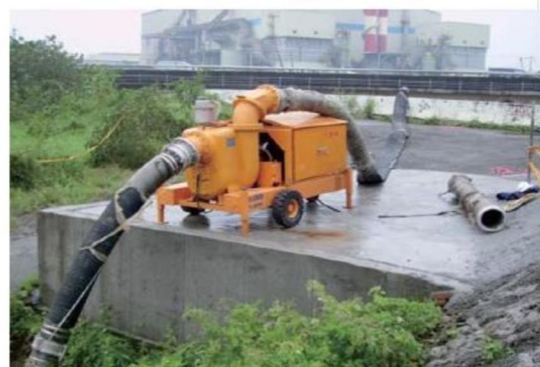
Flood water drainage promptly
