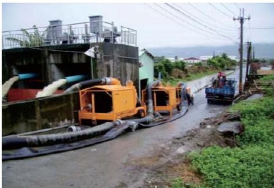
Flood water drainage promptly
