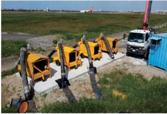
Pump rental at airport
