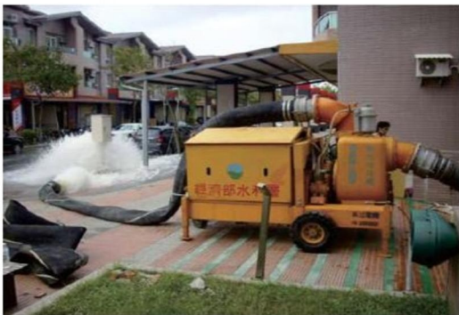
Draining water at basement
