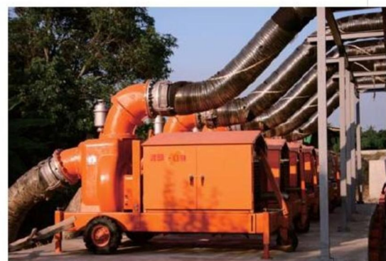
Small pumping station
